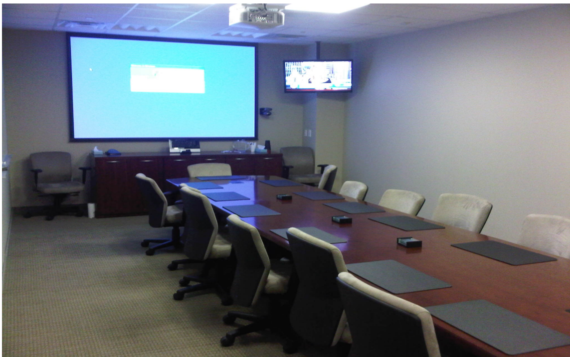
Video conferencing integrated room. Room contains a codec and pan-tilt-zoom camera for video conferencing, touch control panel, LCD display, ceiling mounted microphones, and a projector and screen.
