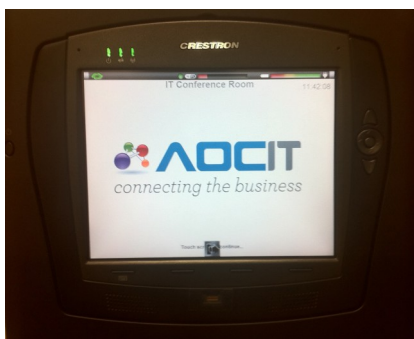
Custom programmed control panel for conference room shown above.
